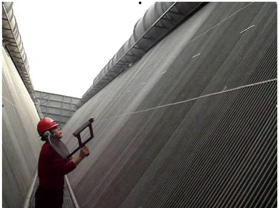
Figure 2. Ultrasound Leak Detection of Condenser
